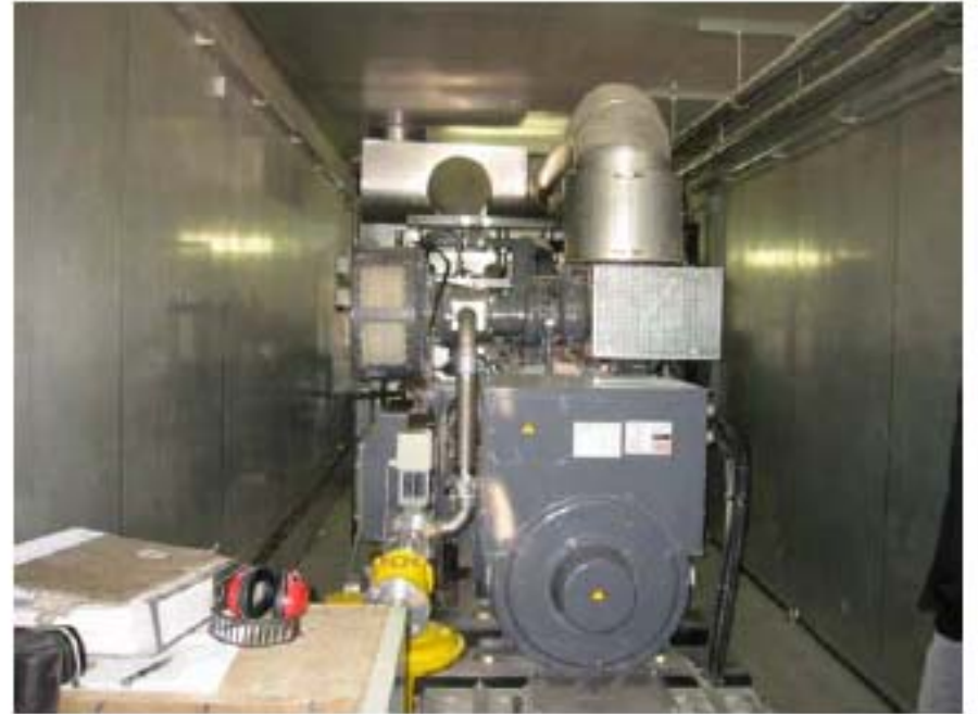
CHP unit within the container
