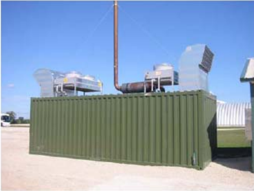
Container housing the CHP unit
